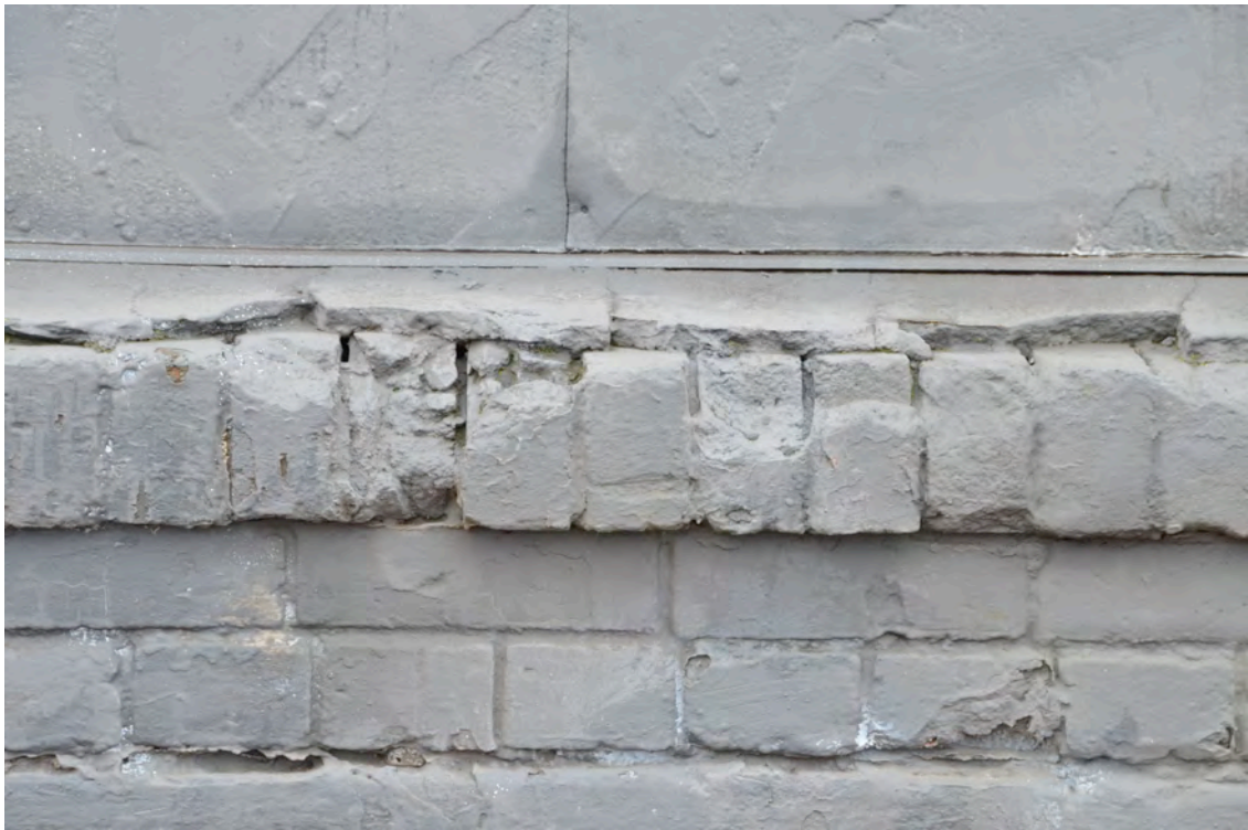
Photo 18 – Rear Façade Showing Condition of Brick Sill and Cap
