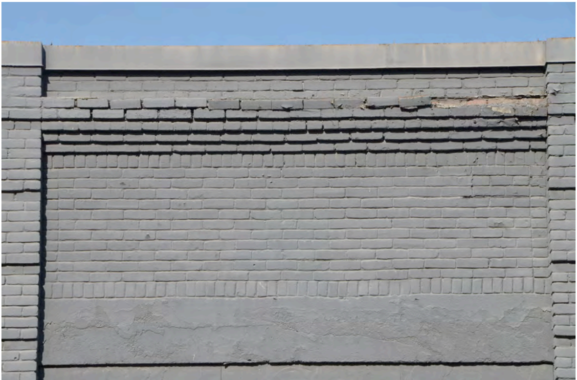
Photo 20 – East Façade Parapet Showing Condition of Brick and Sheet Metal Coping
