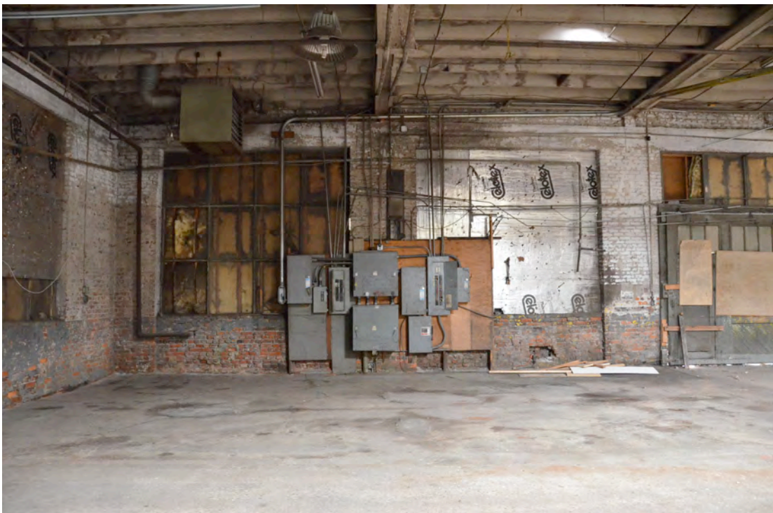
Photo 12 – Looking East Toward NE Corner, Bays 9 & 8, and Electrical Panel
