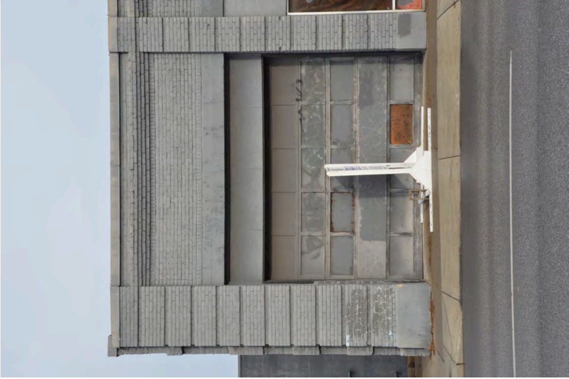
Photo 10 – Front Garage Door-Wood/glass Roll-up
