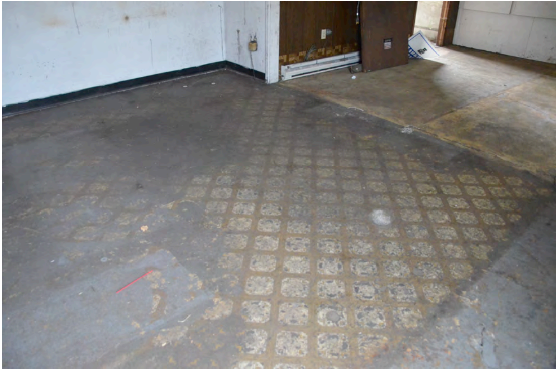
Photo 17 – Looking at Condition of Office Floor – Linoleum over Terrazzo
