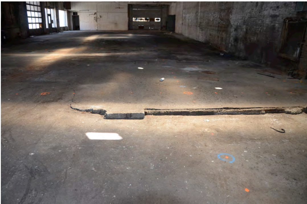
Photo 16 – Looking South Across Garage Showing Condition of Concrete Floor
