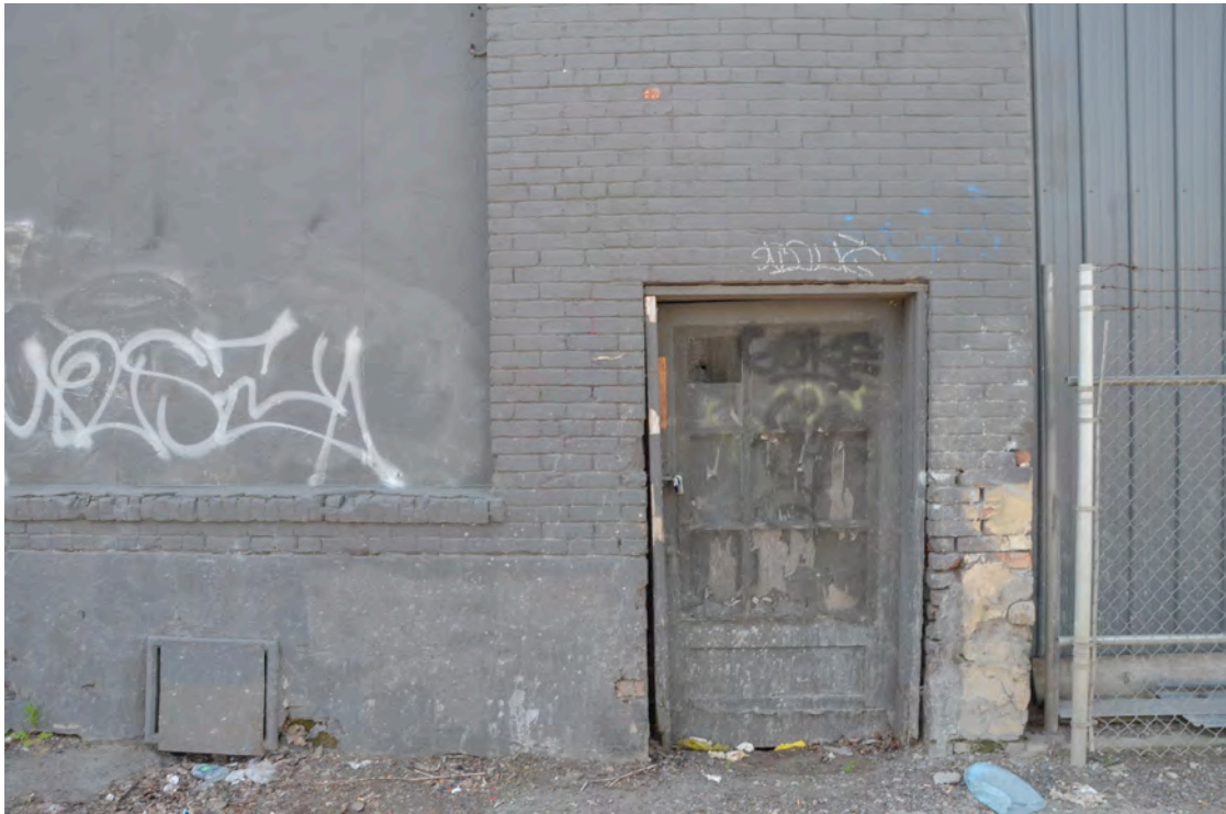
Photo 17 – North Façade –Detail of NW Corner: Pedestrian Door, Window Sill, Brick Condition
