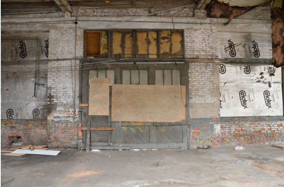
Photo 13 – Looking East Toward Bays 8, 7, & 6 Showing Condition of Garage Door
