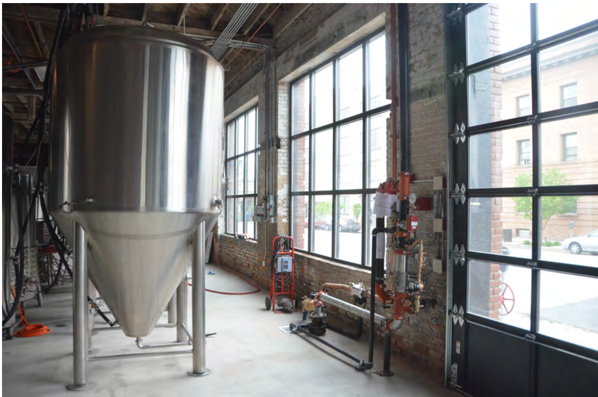
Photo 12 – Looking NE Toward Bays 4, 5, 6 Showing Refurbished Windows and Replaced Rollup Truck Door
