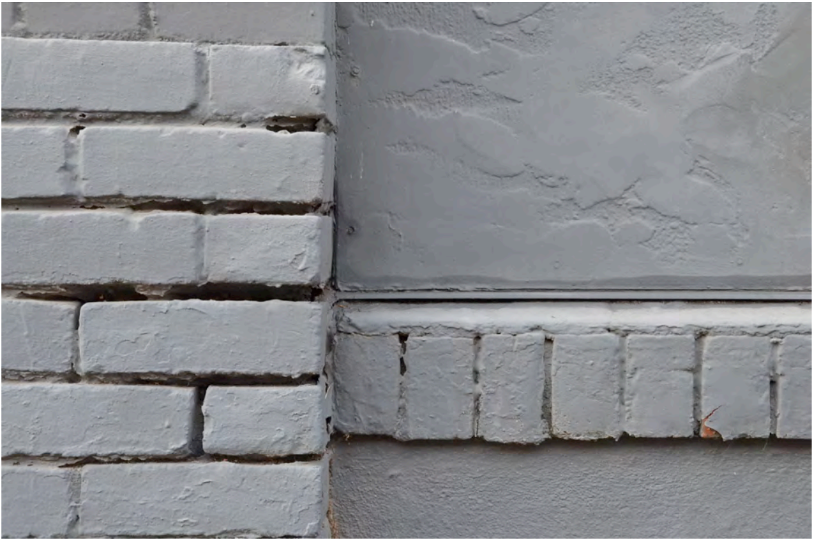
Photo 19 – East Façade Window Bay Showing Deteriorated Mortar Joints
