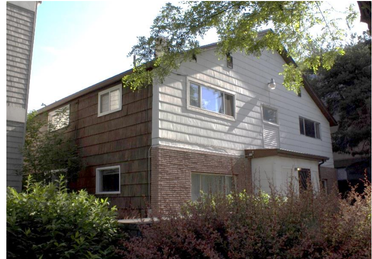
The siding on 1629 W Riverside Avenue has been replaced with non-period appropriate materials for its era of construction.
